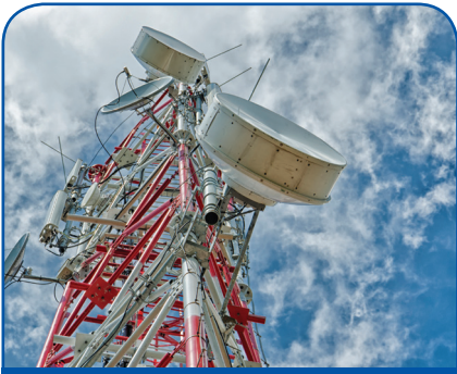
Telecom -Data Infrastructure
