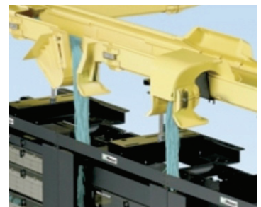
Figure 4.5-4. Example installation of FiberRunner® overhead pathway showing transition to 4-post racks. Cable is 12- fiber jacketed ribbon interconnect.
