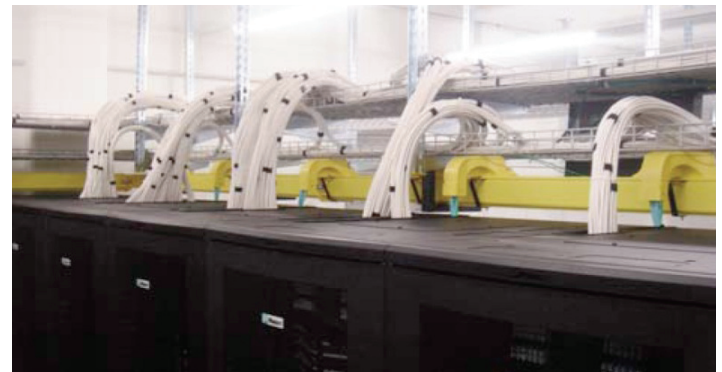
Figure 4.5-5. Example installation of FiberRunner® overhead pathway to PANDUIT® NetAccess™ cabinets. Cable is 12-fiber trunk. Note copper cabling installed in wire basket above FiberRunner® pathway system.
