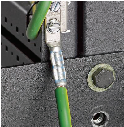
Figure 4.3-11. Grounding washers can be used to create electrical continuity in racks and cabinets. In this photo a bolt and washer is removed, showing paint removal from the contact area (bottom right).
