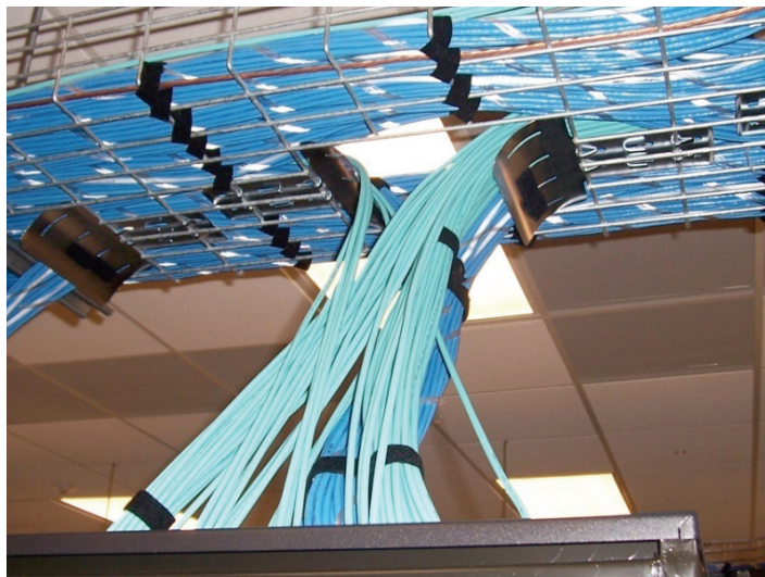
Figure 4.5-10. Overhead wire basket to four-post rack transition.
